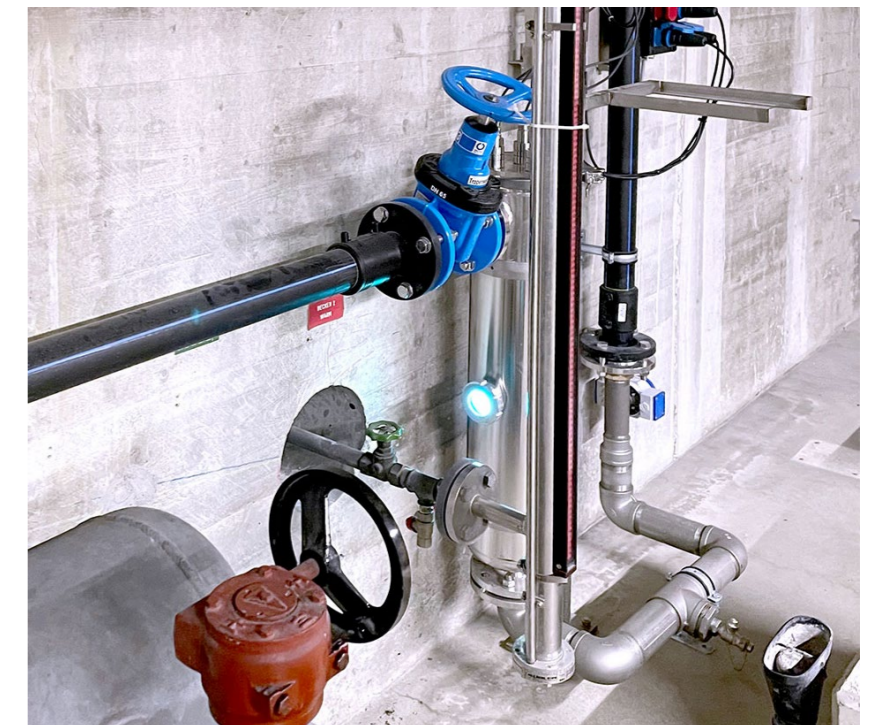
Just two months after the installation of the AQD-ST, water samples showed a significant reduction in the bacterial load of the recooling water.
