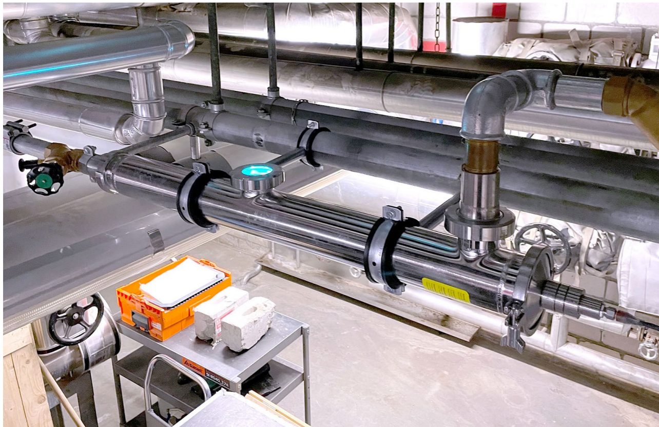
The commissioning of sterilAir UVC devices showed a positive effect after a short time: the bacterial load gradually decreased.
